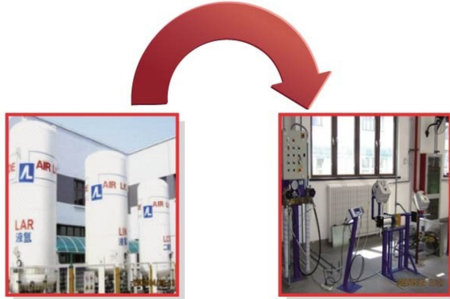
灭火剂储罐 (氩气、氮气、CO2) Gas tanks (Nitrogen, Argon, CO2)
